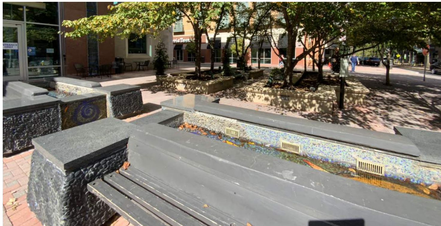
Inoperable fountain at library plaza.
